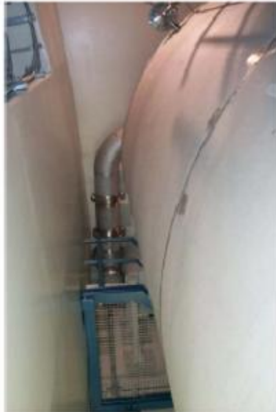
Filter room: Clean gas piping (bottom up view)
