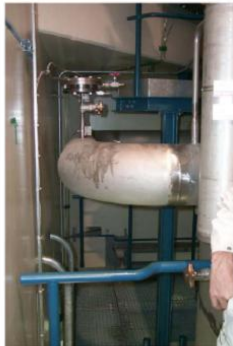
Filter room: Inlet piping
