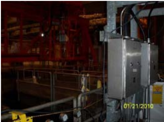
Fig.5.16 FB-113 Fuel Handling Platform
