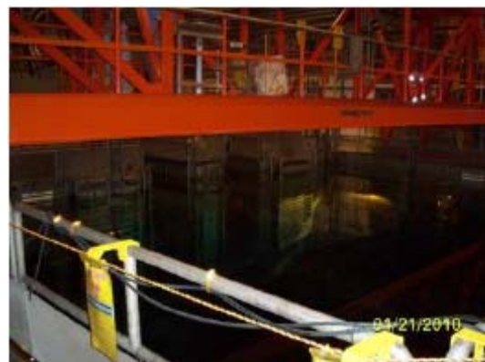
Fig.5.3 FB-113 Spent Fuel Storage Pool (写真左奥側で SHIPPING 検査を実施中)
