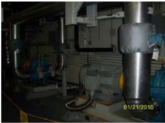
Fig.5.11 Suppression Pool Cooling Pump
