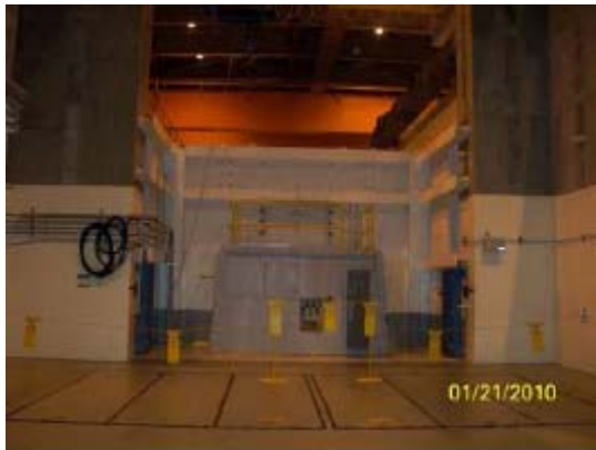
Fig.5.22 TB-123 Turbine Front
