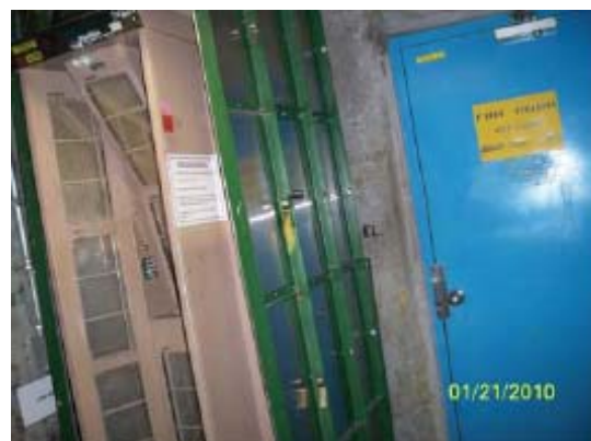
Fig.5.6 In Plant Personnel Contamination Monitor
