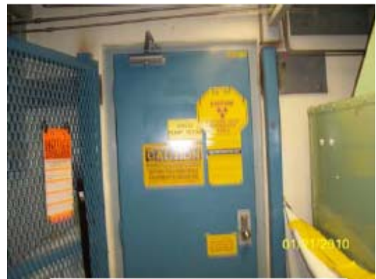
Fig.5.8 RWCU Pump Room
