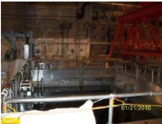
Fig.5.18 FB-113 Cask Handling Pool
